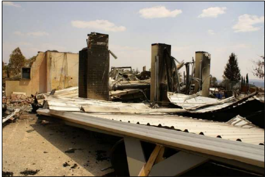
Figure: A fully burned house
